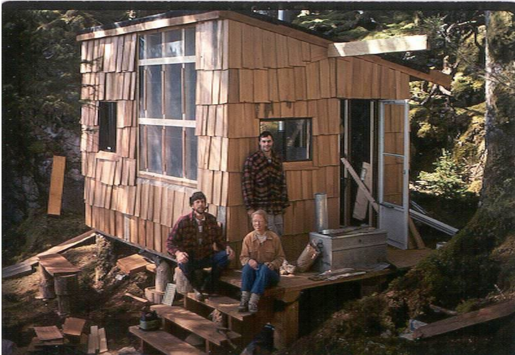
Work party building the original cabin on East Limestone in May of 1990
